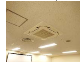
Individualized air-conditioner in B1 floor (Osaka Nakanoshima Building)
